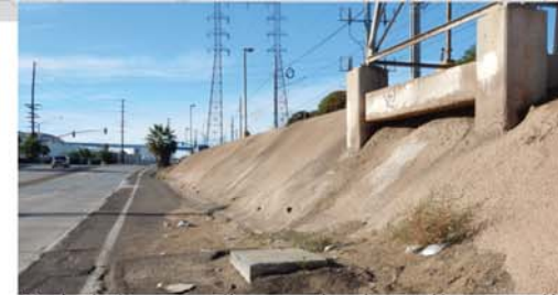
Retaining wall needed on the north side of harbor (photo looking north).
