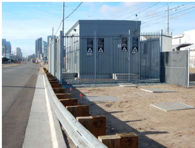
Figure 26: The addition of this power substation creates an obstacle within the ROW.
