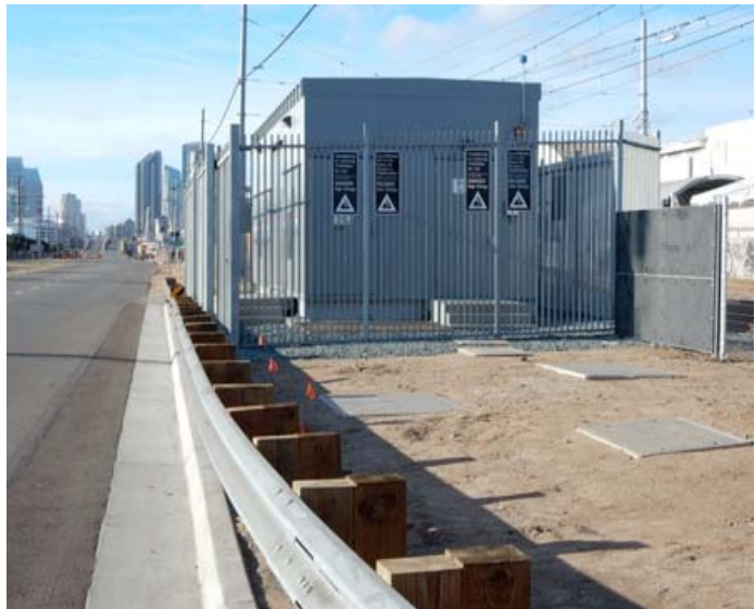
Figure 19 - Bikeway needs to be routed around MTS power station
