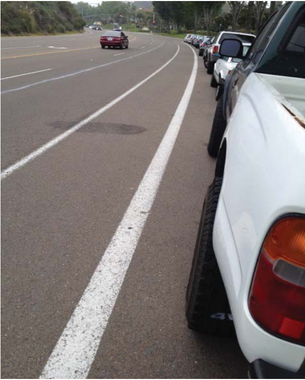
Gilman Drive in La Jolla - note the excellent clean smooth road surface for safety
