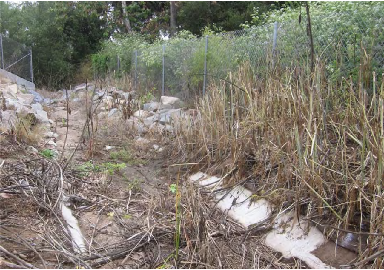
Photograph 13. North of the NCTD rail, representative proposed jurisdictional concrete lined drainage ditch; ditch drains to Buena Creek.
