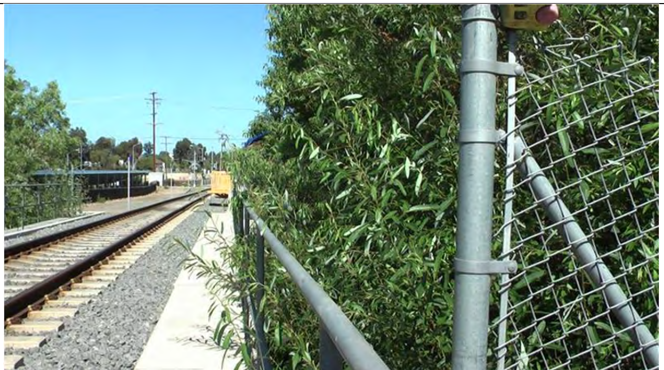
Photo 4j. Looking west from northeast side of bridge. Vegetation is SAWRF on the north and too dense to see all the SCLORF habitat that begins only about 50 feet north of the bridge.
