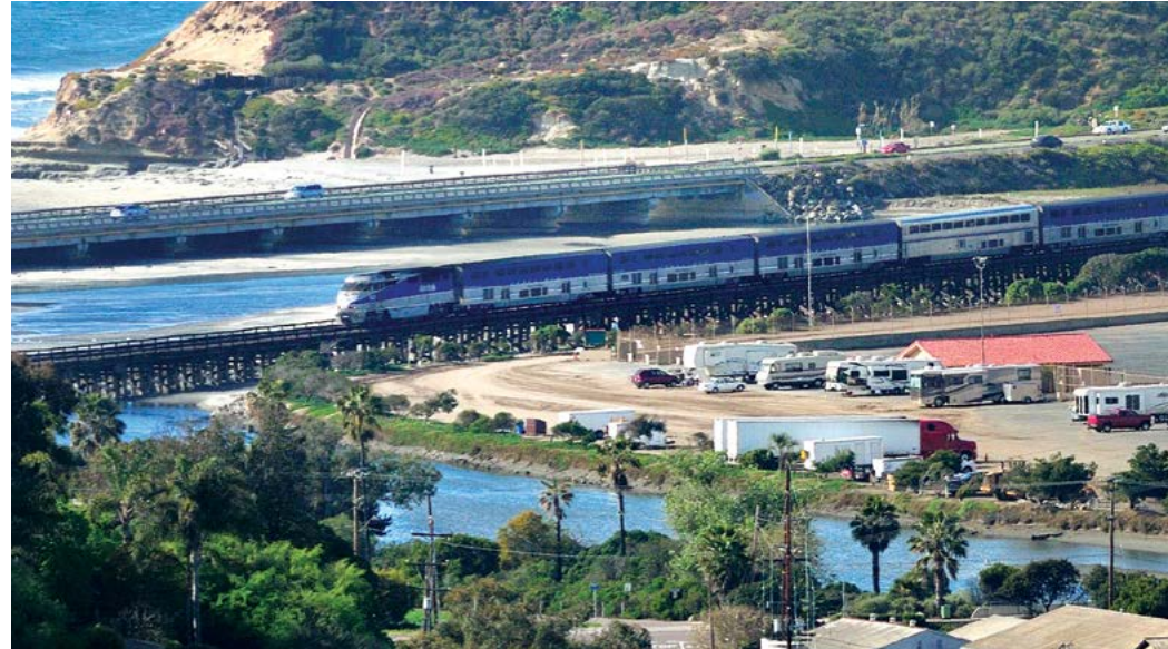
The existing 97-year-old wooden-trestle rail bridge over the San Dieguito River and Lagoon will be replaced with a modern, concrete bridge, resulting in a quieter ride for passengers and potentially reducing noise for adjacent residents.
