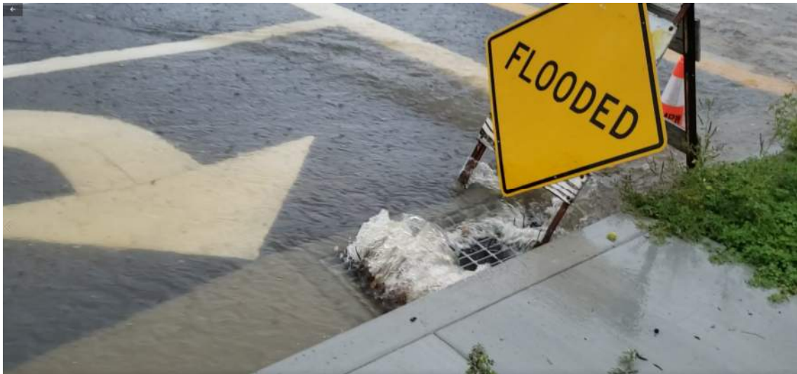
Figure 3. Inlet Bypass at the Intersection of 9 th Street and Camino Del Mar
