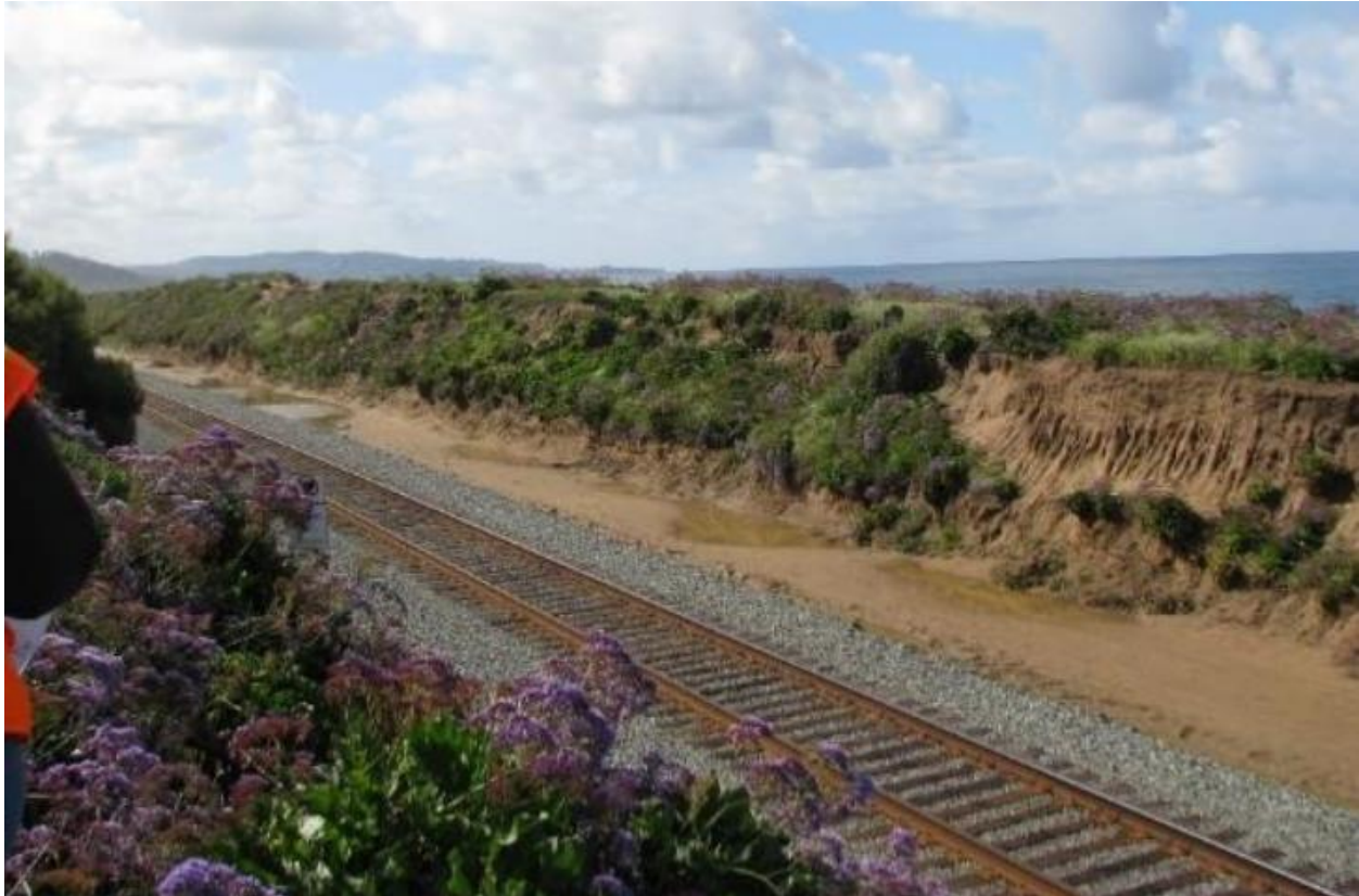
Figure 30 – Photo of Existing Ponding between Track and Beach
