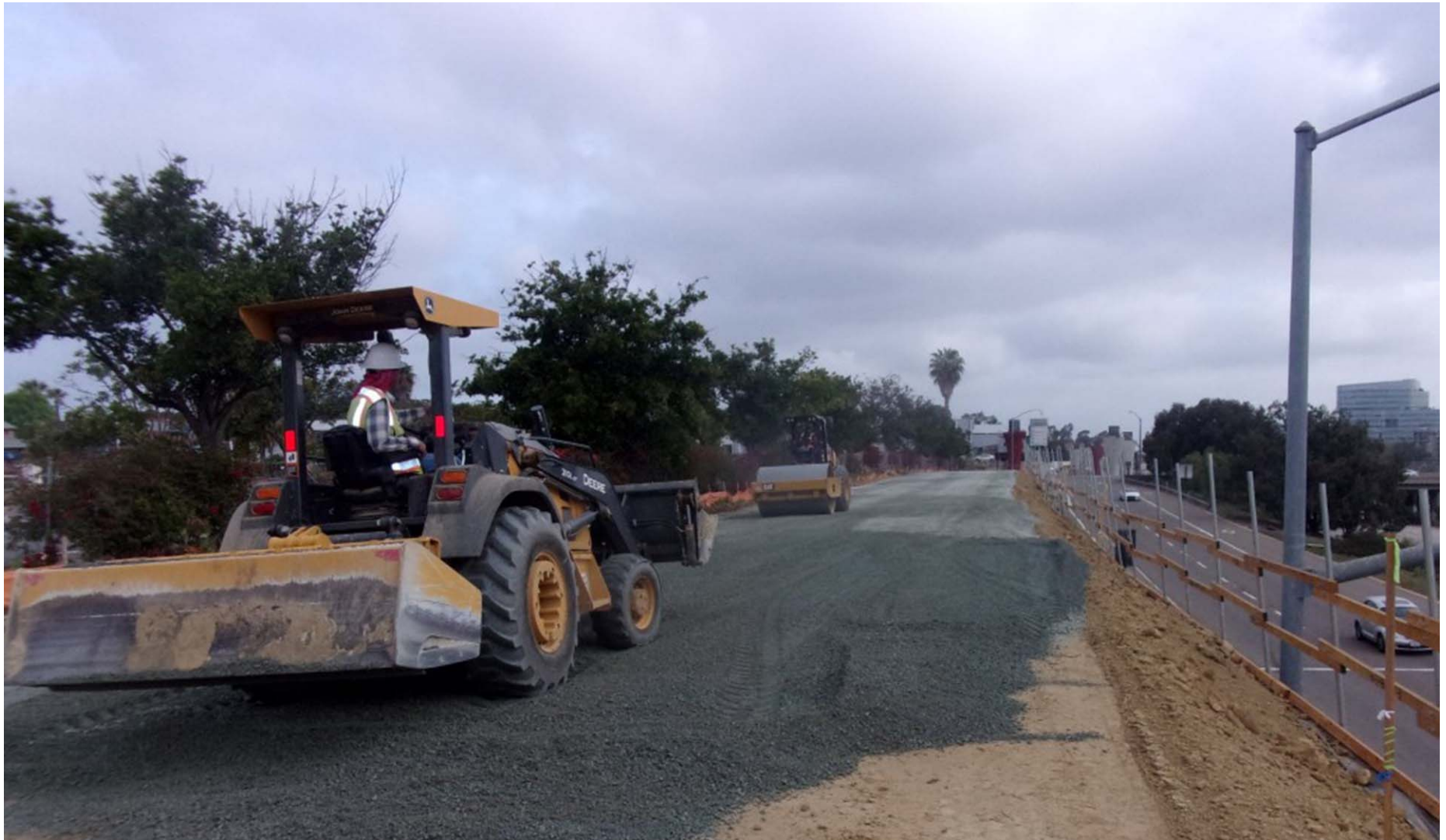
Southbound I-5 Nobel on-ramp Temporary wire wall and grading Construction (looking north)
