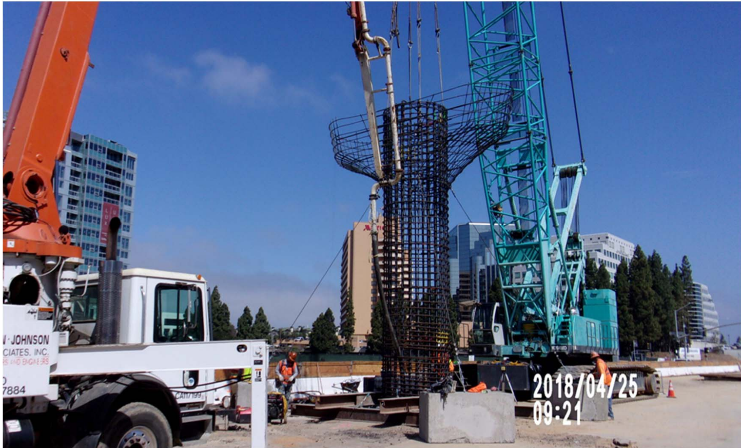
Pouring Genesee Viaduct CIDH at Bent # 25 (looking north towards La Jolla Village Dr)
