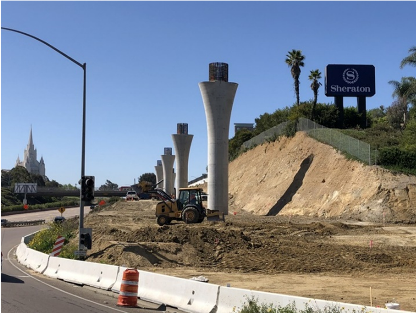
Nobel Viaduct Falsework pad grading for Frame 9 (looking south on LJVD on-ramp)
