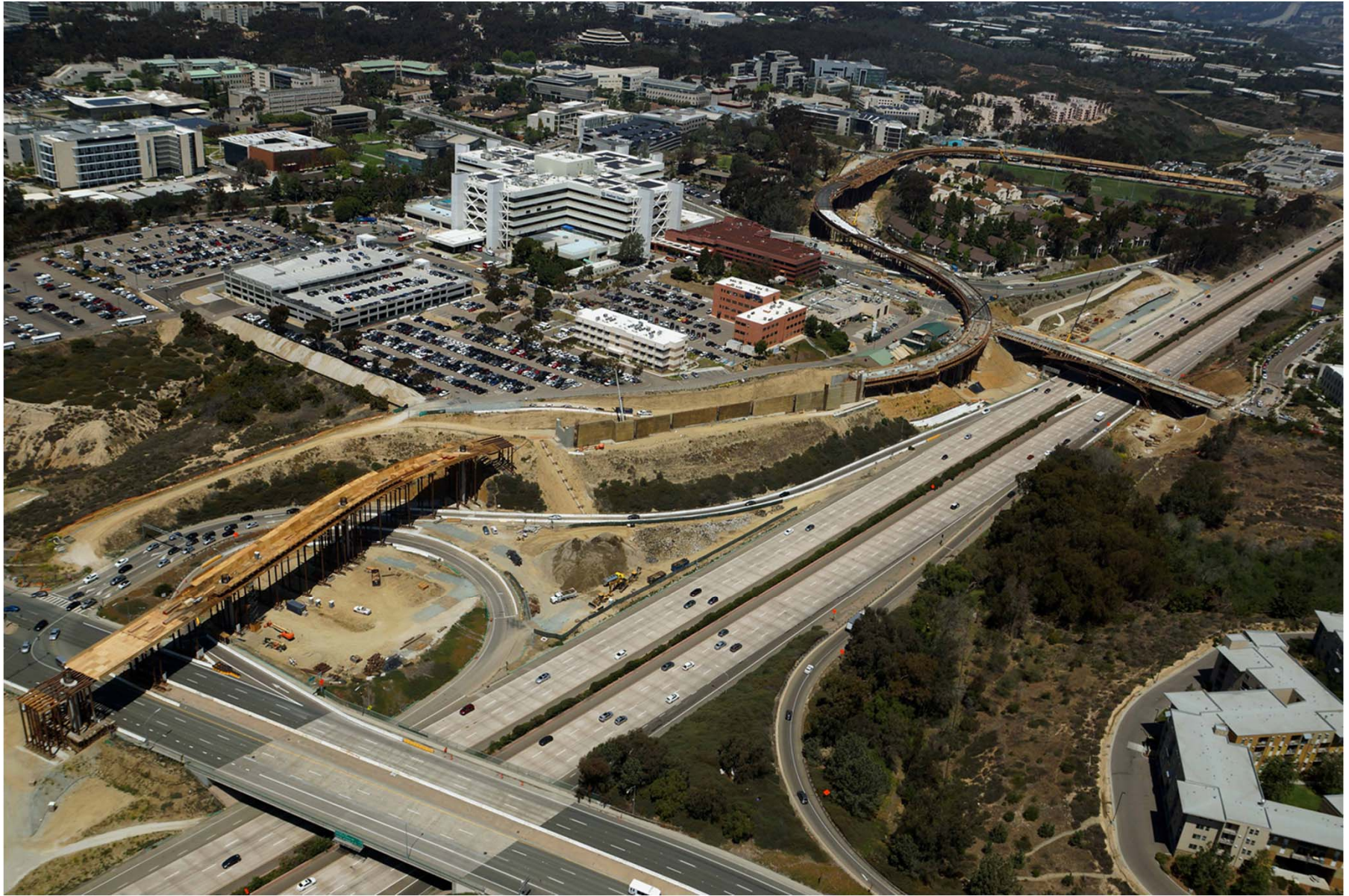
Looking Northwest at La Jolla Village Dr towards VA Medical Center Station
