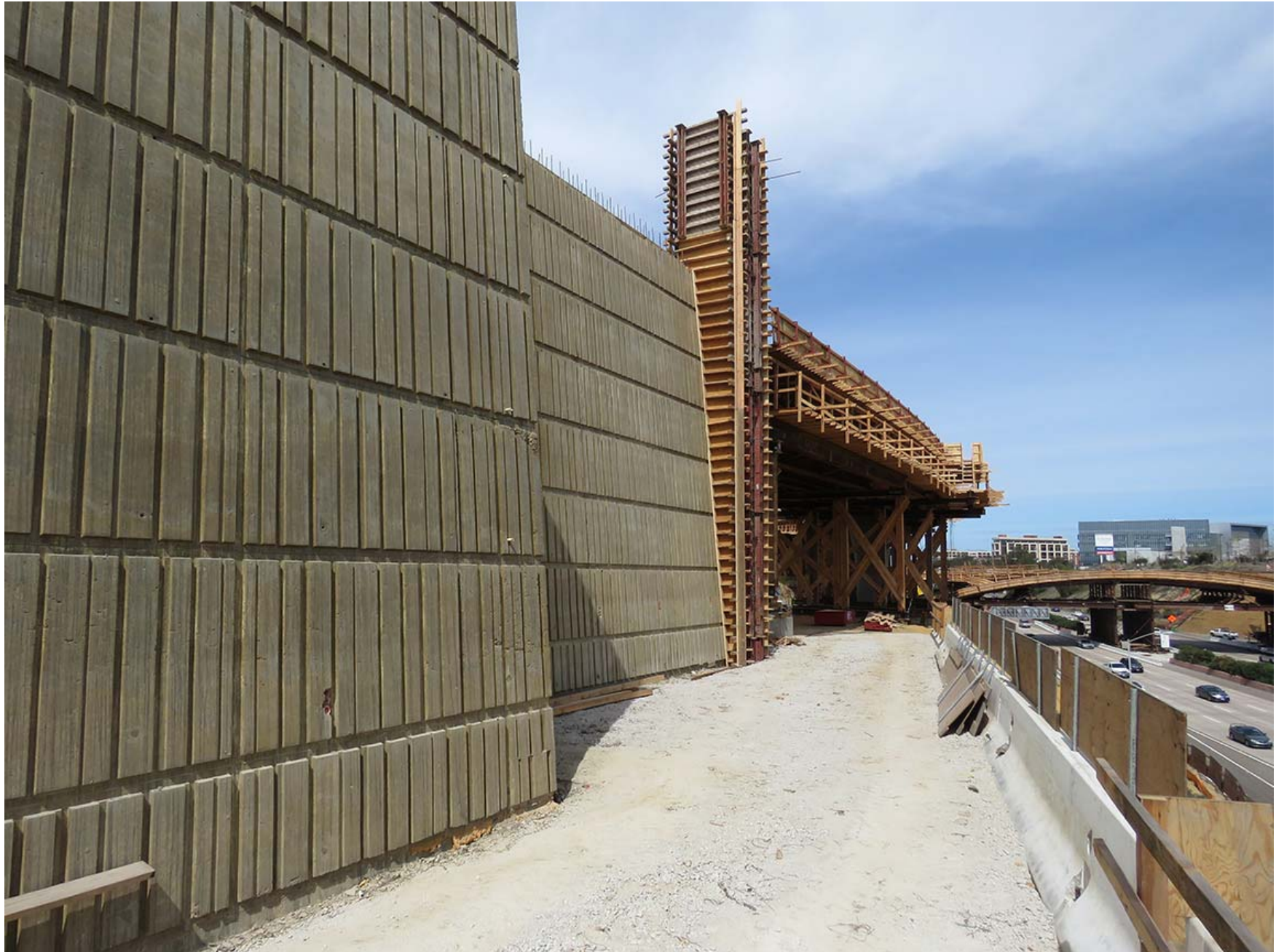
Looking North at VA Medical Center Station With the Gilman Bridge in background
