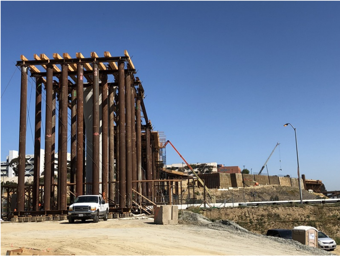
Looking north at falsework over La Jolla Village Drive (RW 848 in background)
