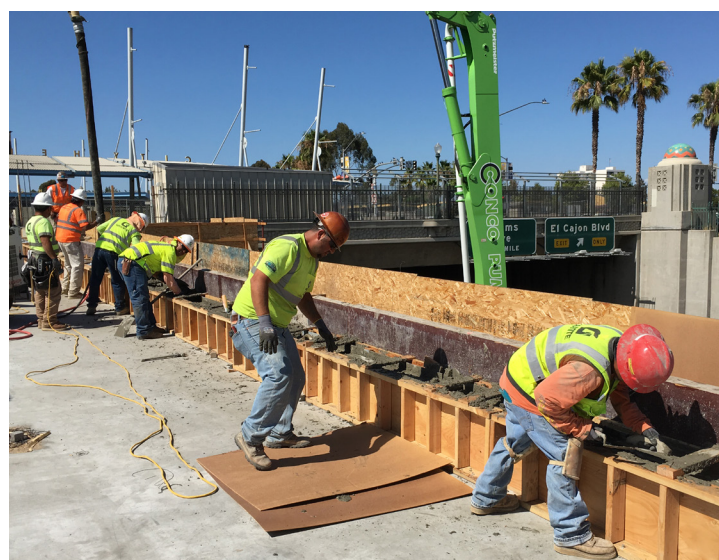
Construction crews form the curb that will align the pedestrian bridge in the SR 15 median south of University Avenue.
