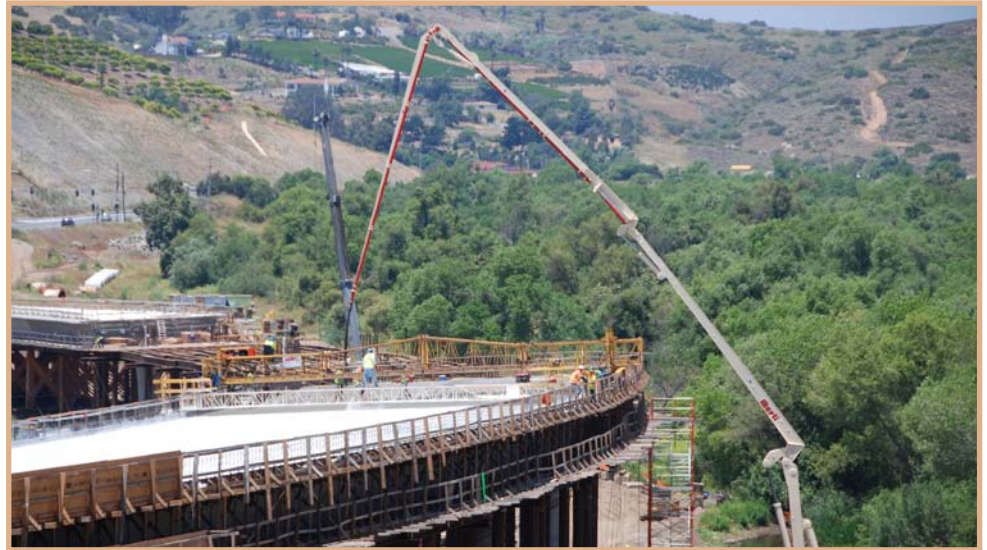
Crews poured concrete for the deck of the west section of the San Luis Rey bridge structure.
