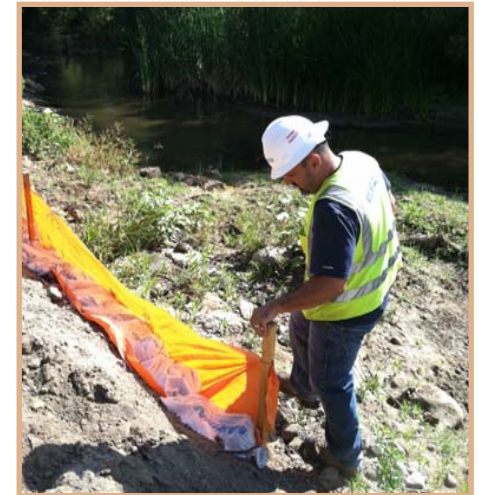
Ruben Ramirez erecting a fence to keep arroyo toads out of the project site.
