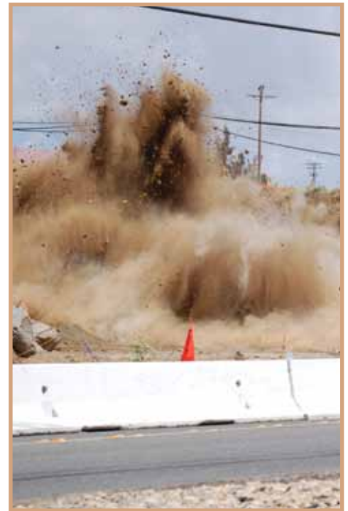
Photo of recent bedrock blasting that took place on North River Road.
