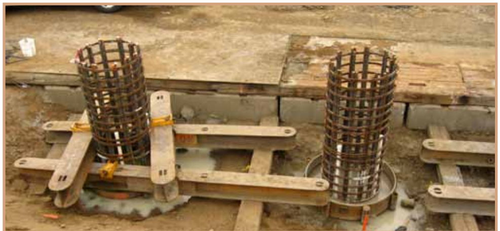
Photo of rebar support columns that will be up to 10 feet in diameter for the new bridge over the San Luis Rey River. Motorists will begin to see the columns from the highway this summer.
