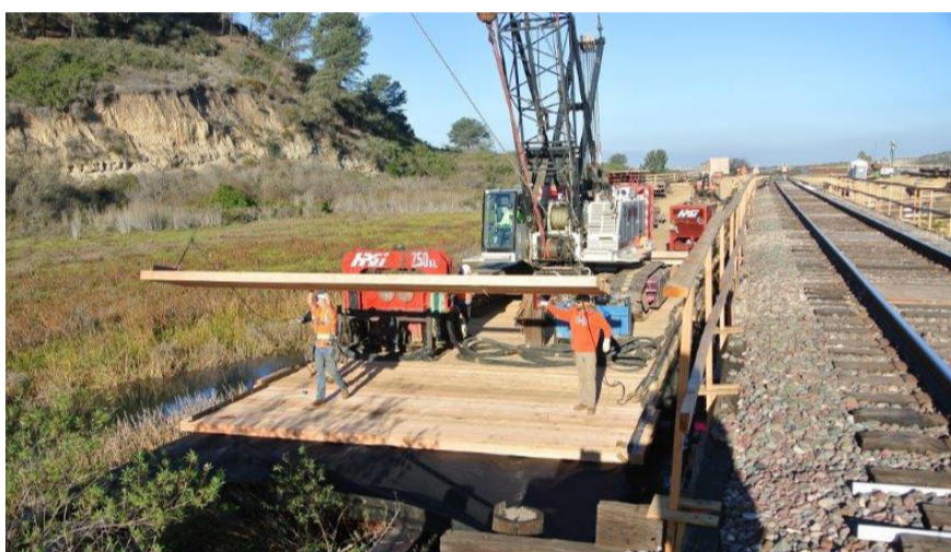
A temporary structure is being constructed on one of the center bridges. It will be used as a platform for machinery and to stage/move materials to build the new rail bridge.
