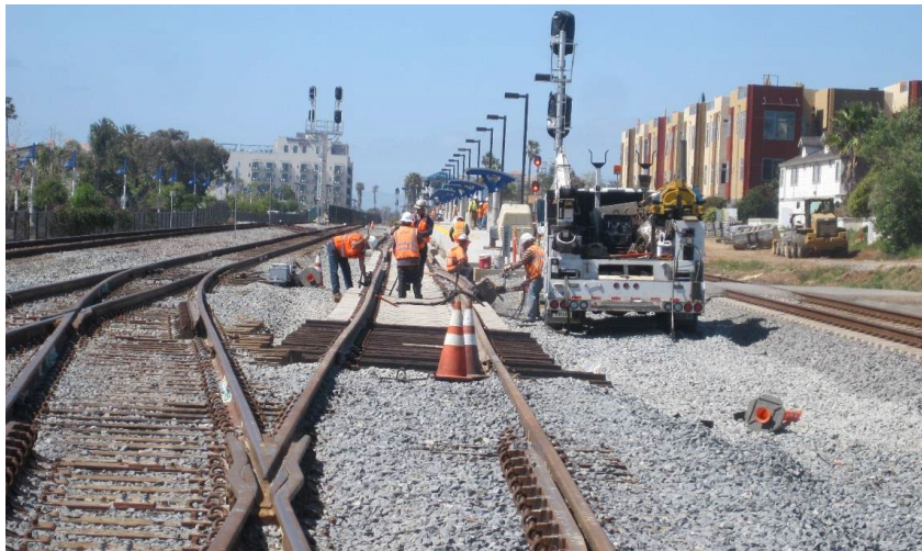
Crews work on the new third track south of the Oceanside Transit Center.
