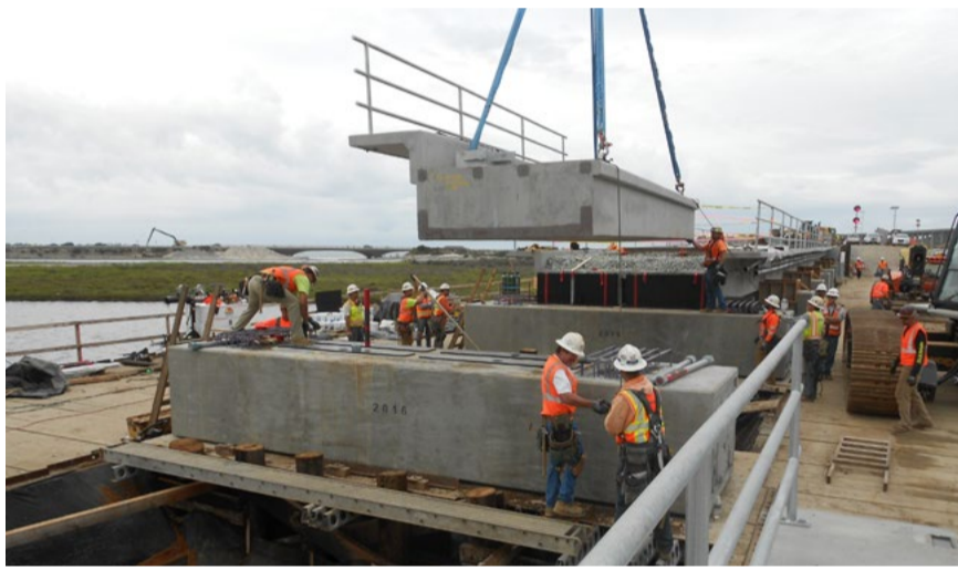
Crews have made significant progress on the bridge construction, and the project is expected to be completed in early 2017.
