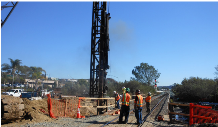
Crews drive the last of the bridge piles at the southernmost rail bridge.
