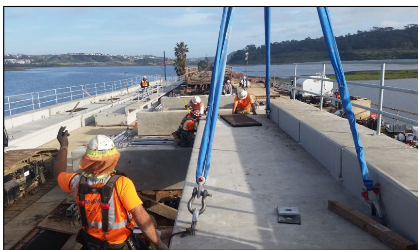
Crews place the precast concrete bridge girders of the new northernmost bridge during an AWW.
