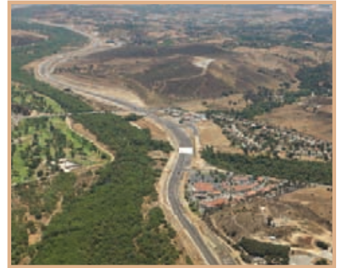
Looking west at the improved SR 76 Middle Segment, which is nearing completion.
