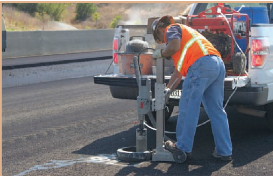
A crew member coring the pavement on the SR 76 westbound lanes to assess the condition of the surface prior to laying new pavement.
