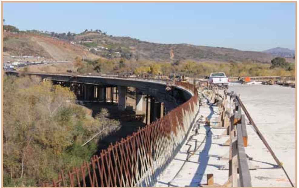
Crews work to complete the San Luis Rey River bridge structure by March 2012.
