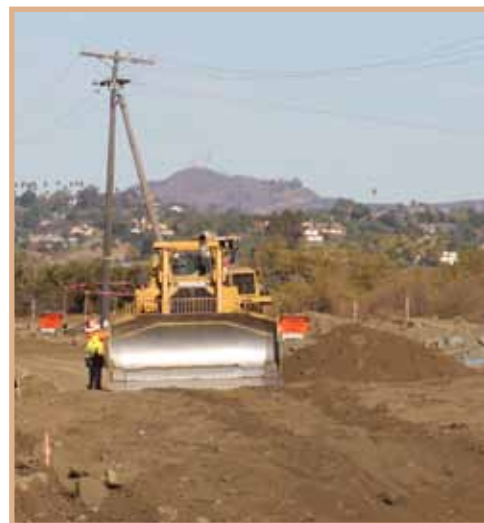
Crews move and compact soil to build a foundation for the new highway.
