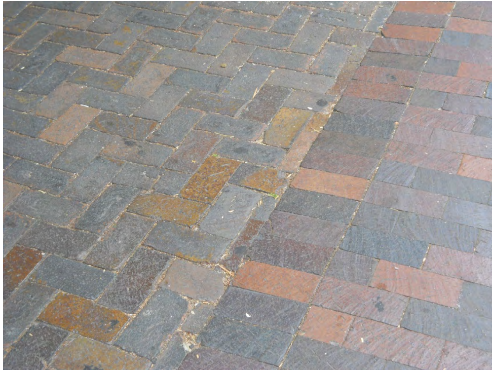
Klinker bricks (on left) adjoin new brick
