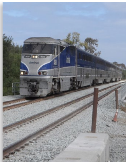
The project added one mile of new double track north of the Sorrento Valley COASTER Station.
