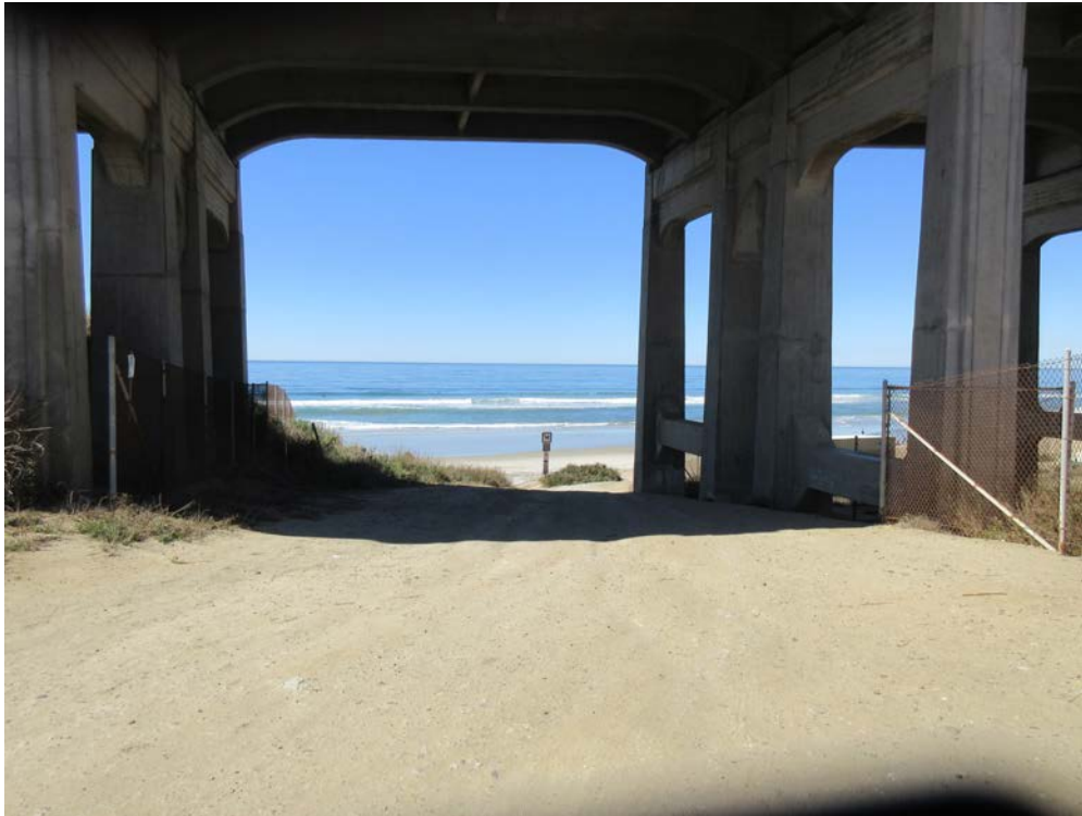
Photo 13. Looking west at the southerly beach access route where it crosses below North Torrey Pines Road bridge.
