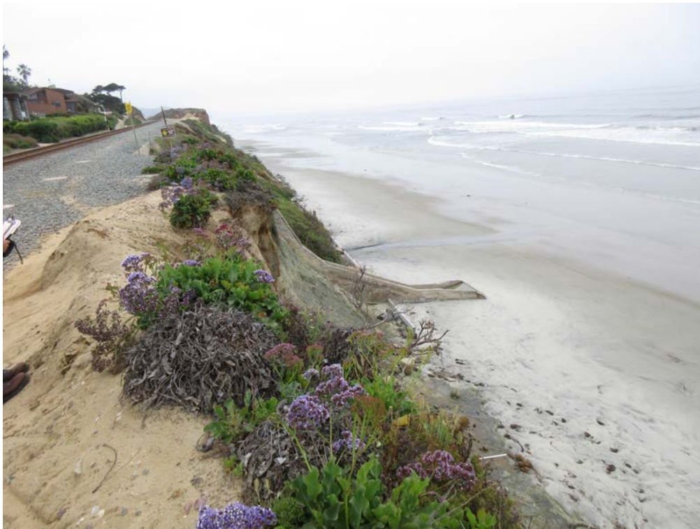
Photo 4. Looking south at disturbed bluff and a concrete storm water outlet onto the beach in the northern part of the study area.
