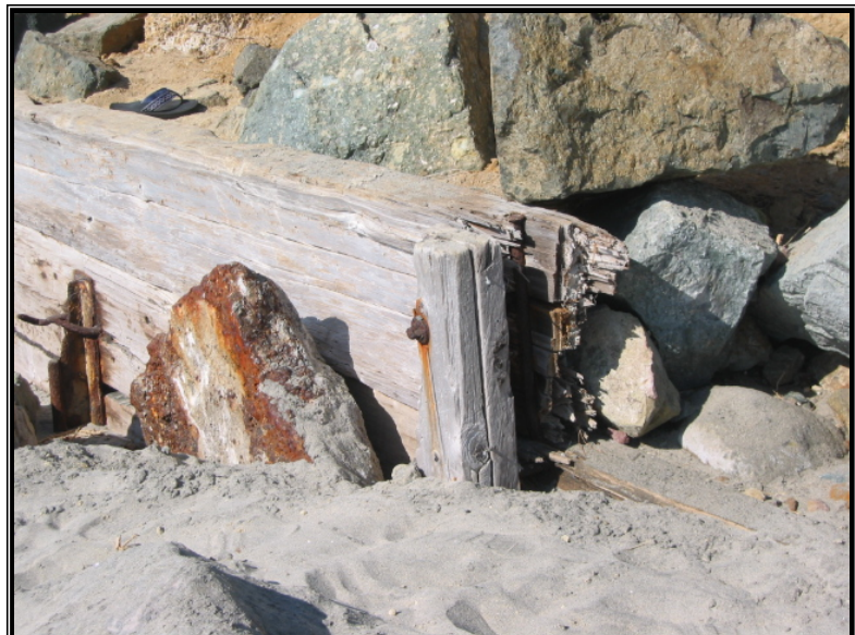
Figure 10. Failure of Timber Wall Extension
