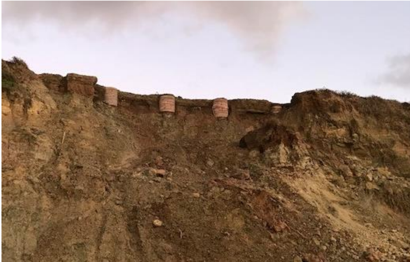
Damage before repair was completed – Piles supporting track bed
