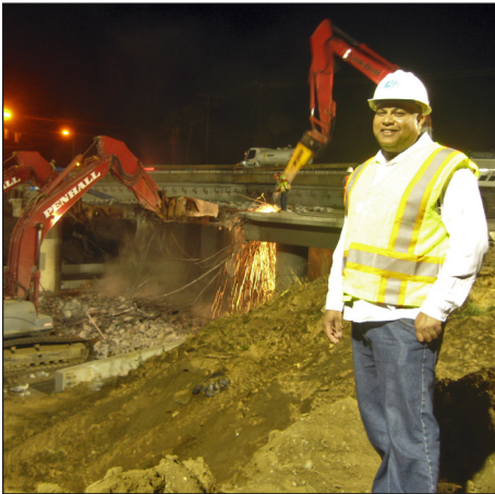
August 2012 - Senior Resident Engineer Faridun Javed overseeing the demolition of the Nordahl Road bridge's west side.
