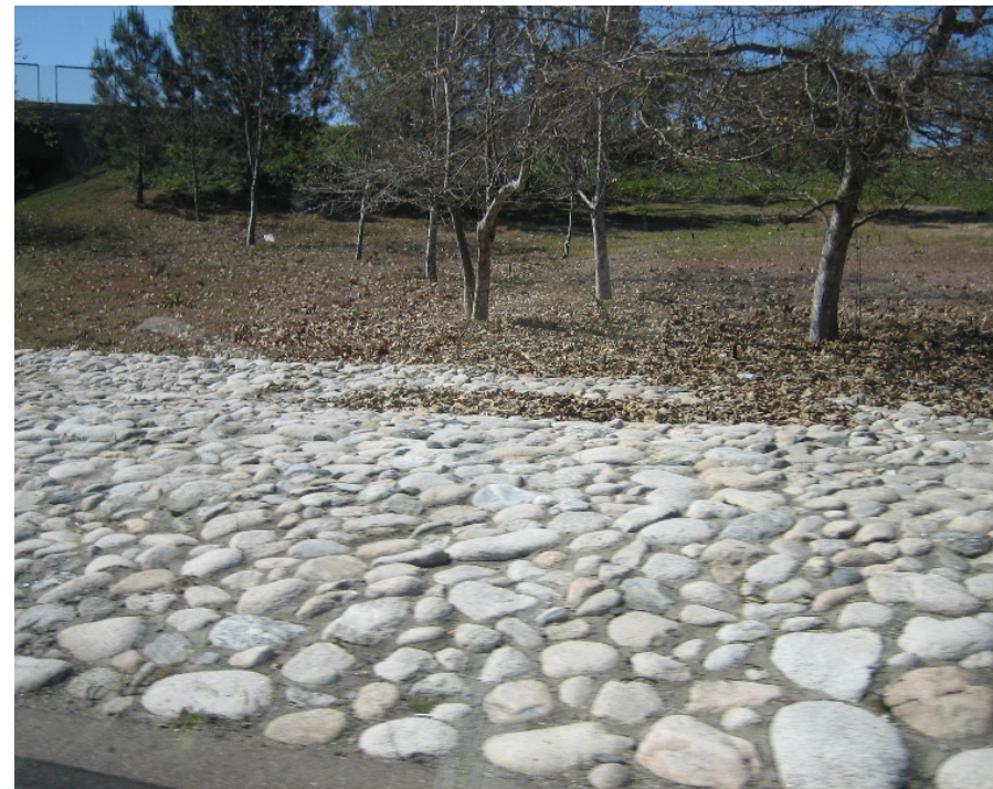
Rounded creek cobble could be used where possible for slope paving under the bridge structures and in areas of the project that are too shady to plant
