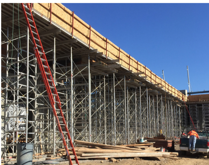
Great progress has been made on the deck of the pedestrian bridge in the SR 15 median south of University Avenue.
