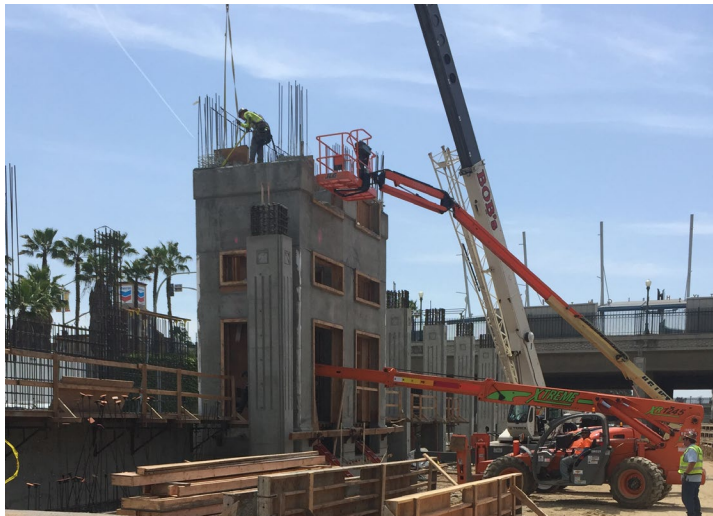
Crews work to form and pave the elevator building north of University Ave.
