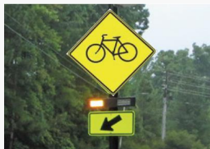
Rectangular Rapid Flashing Beacon
