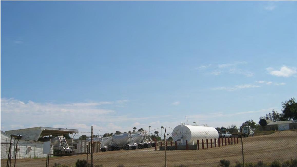
View of 10,000-gallon above ground fuel tank at South Bay Salt Works maintenance yard located on the east side of Bay Boulevard, accross from the entrance to the main facility
