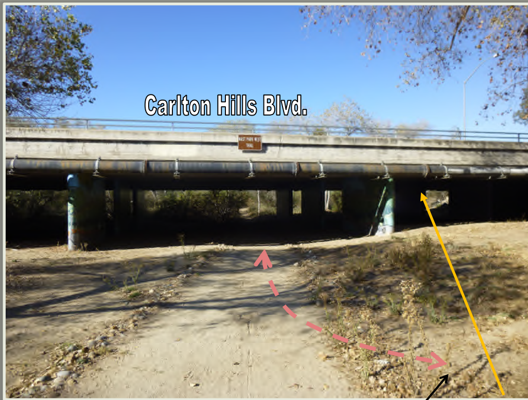
Photograph 27: Viewing west where the bikeway path will extend under Carlton Hills Boulevard.
