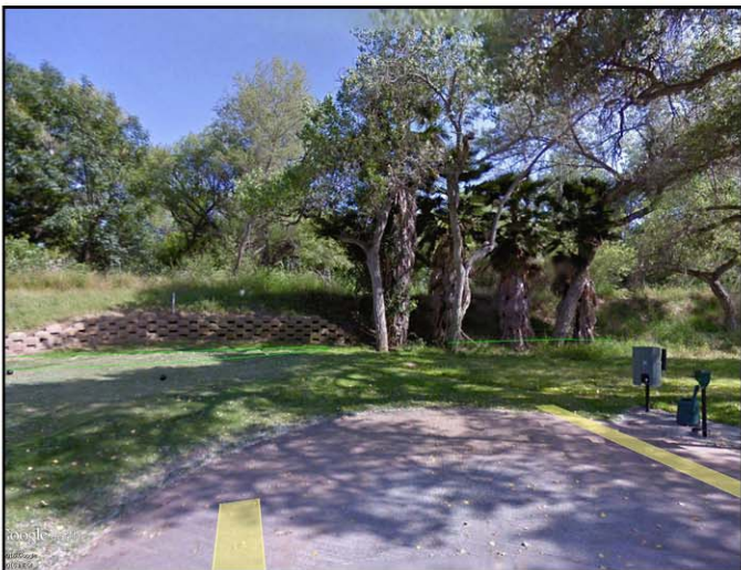
Photograph 9: Southward toward the existing berm and retaining wall at Sixteenth Tee Box
