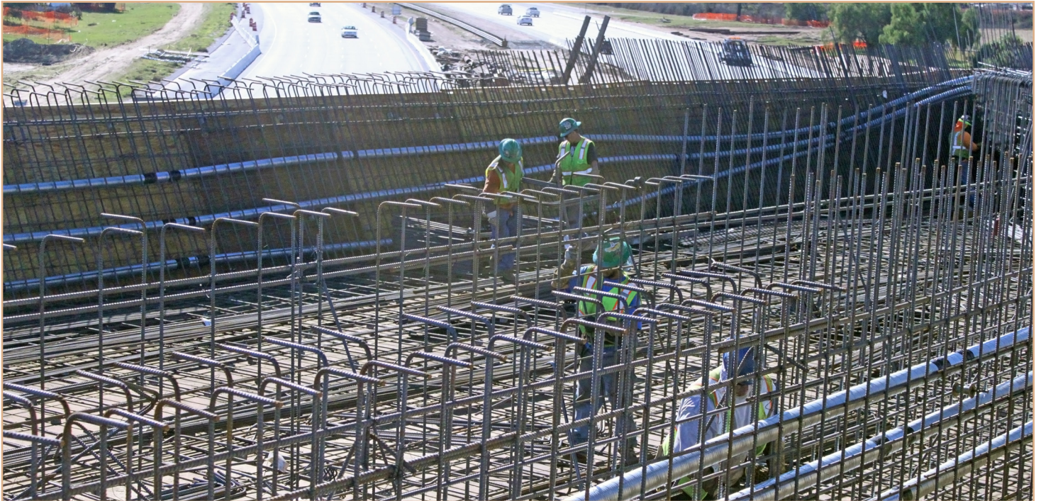
Current construction includes installing rebar (steel bars) to reinforce the structure of the bridge
