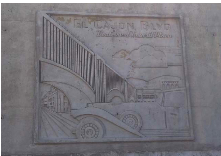
Crews have finished installing the first decorative relief panel along transit station walls at El Cajon Boulevard.
