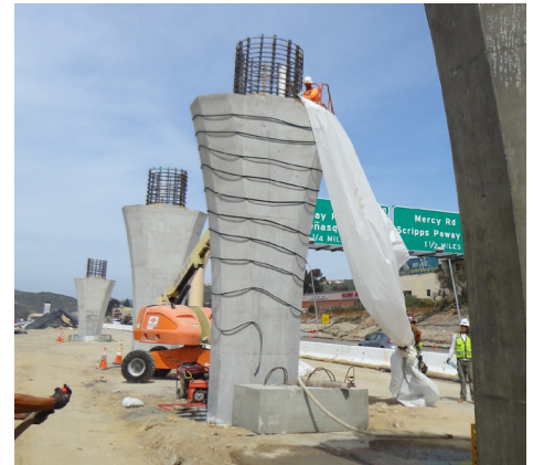
April 2013 - Crews constructing columns that will support the DAR over I-15 in Mira Mesa.
